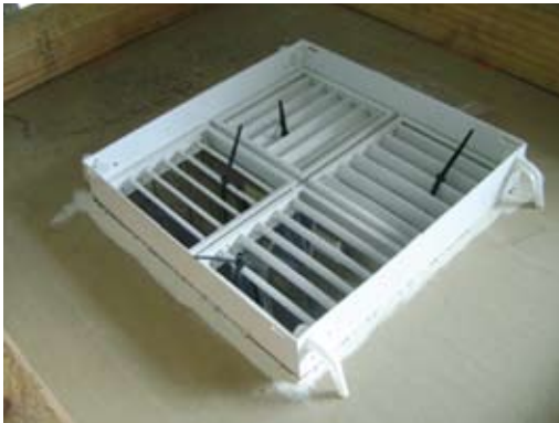
MDO-X attached to ceiling with new clips (Black Cable ties are holding suspended weights)
