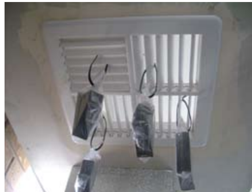
Viewed from underneath showing Suspended weights
